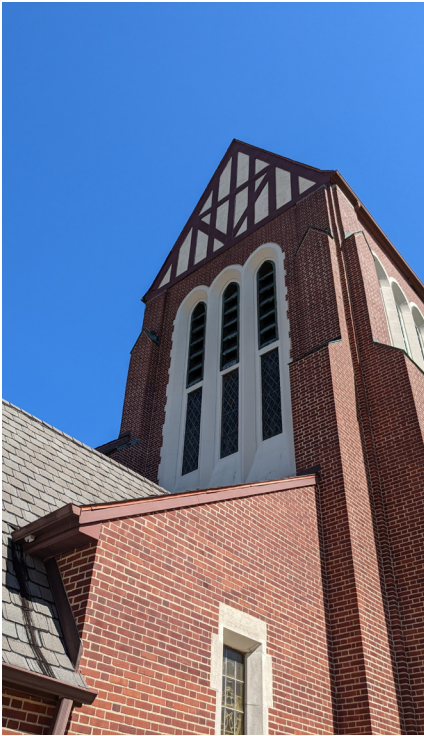
The roof of the church shows evidence of hail damage. The aluminum flashing is also loose.
