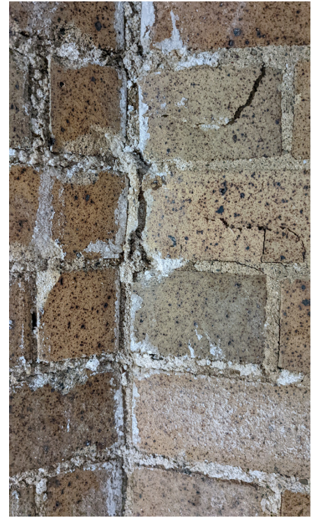
Effervescence can be seen on the bricks inside the turret which houses the spiral staircase that leads to the balcony. This indicates long-term water infiltration.
