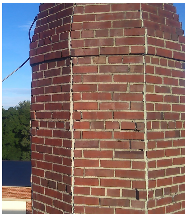
The photo above shows the deterioration of the church chimney that has occurred over the years. It is important to repair the masonry soon, to maintain the integrity of the structure.
